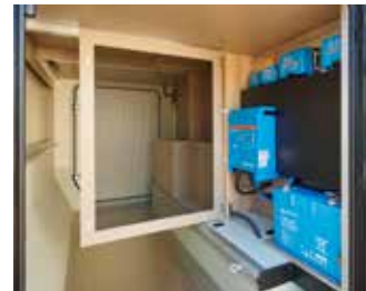
Garage with electrical distributor panel
