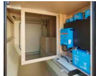
Garage with electrical distributor panel
